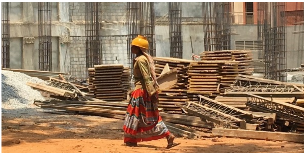
A female worker walking across a large construction site in Bengaluru. Photo credit: Rebecca Bowers.
