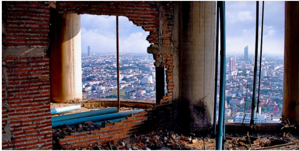
47th floor in the abandoned skyscraper Sathorn Unique Building, Bangkok. Credit: Just One Way Ticket CC BY-NC-ND 2.0
