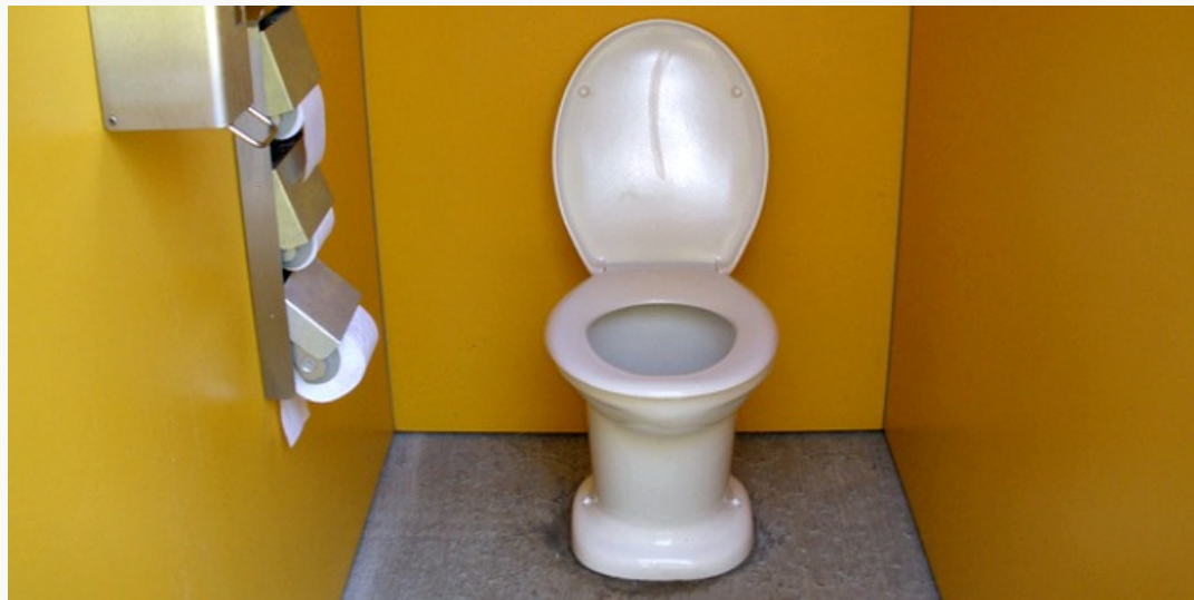
Enviroloo dry toilet top part of the composting system at public toilet in Norderstedt, Germany. Credit: SuSanA Secretariat CC BY 2.0
