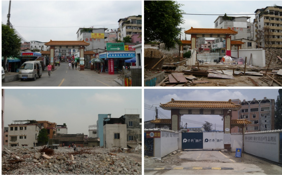
Figure 2: Pazhou in the midst of demolition (Photographs by the author between 2009 and 2011)
