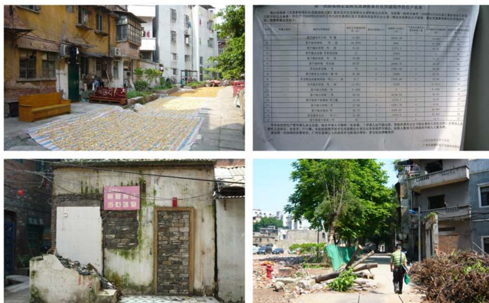
Figure 1: Enning in the midst of demolition (Photographs by the author between 2009 and 2011)
