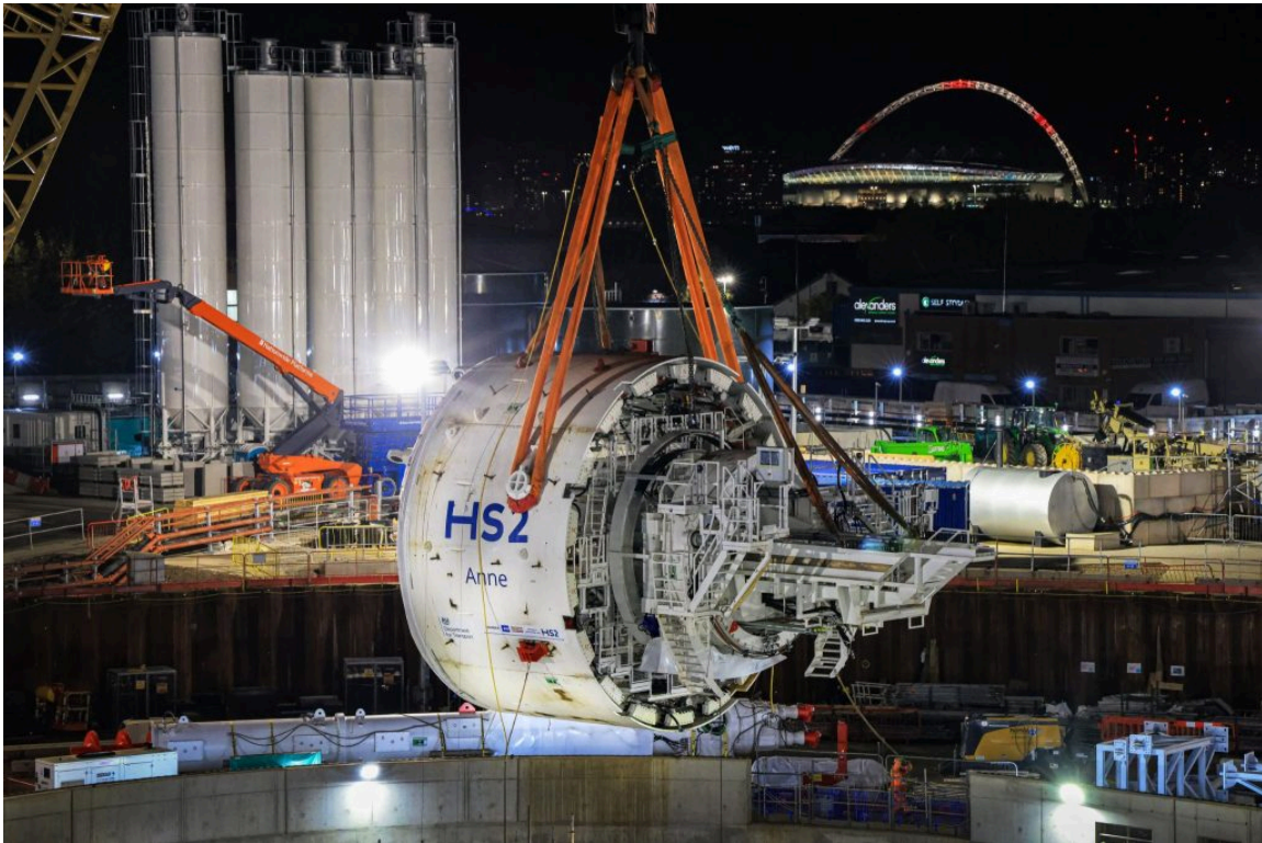
HS2 tunnel boring machine being lowered into launch chamber in West London. Source: HS2 Ltd.
