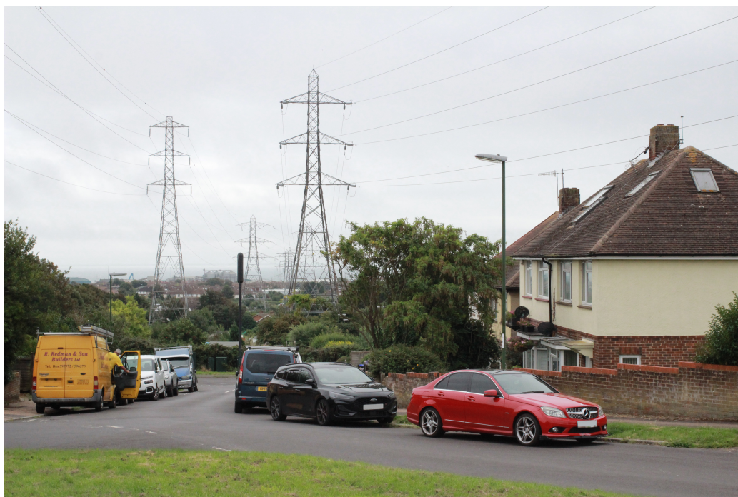
Figure 1: 132kV overhead lines and pylons in a suburban setting in England ©Stephen Gibbons 2023.
