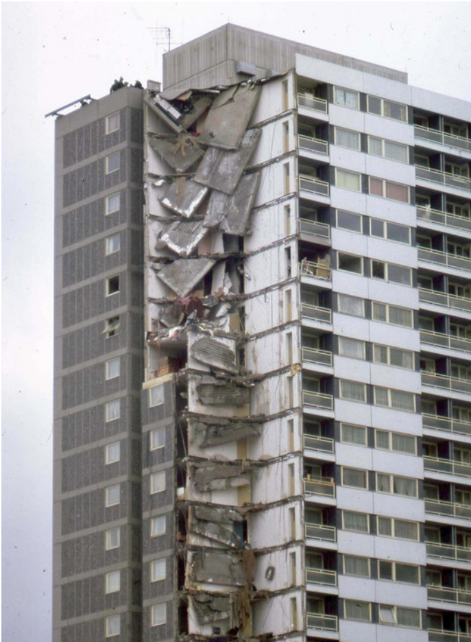
Figure 4.5: Effects of the explosion at Ronan Point tower block on 16 May 1968
