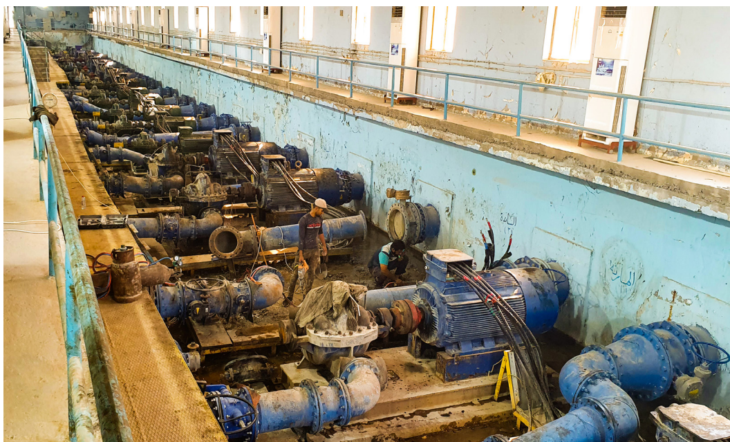
Figure 5: Interior of the R Zero Water Treatment Plant, November 2020.
