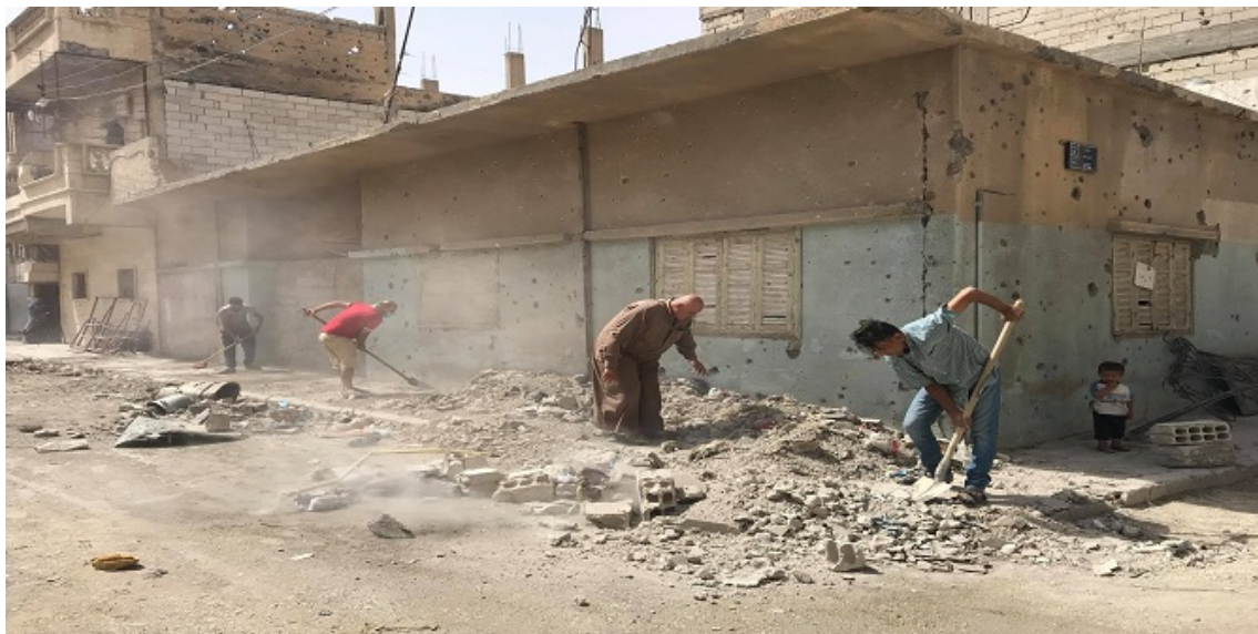
In the absence of reconstruction programmes for their destroyed city, the civilians in Raqqa begin repairing their houses and removing debris from the streets. Credit: Aboud Hamam.
